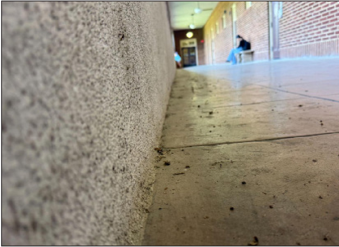
Pieces of dirt and debris on the floor of upstairs in the Old Administration Building hallway, March 26. Photo by Sophia Wilson.
