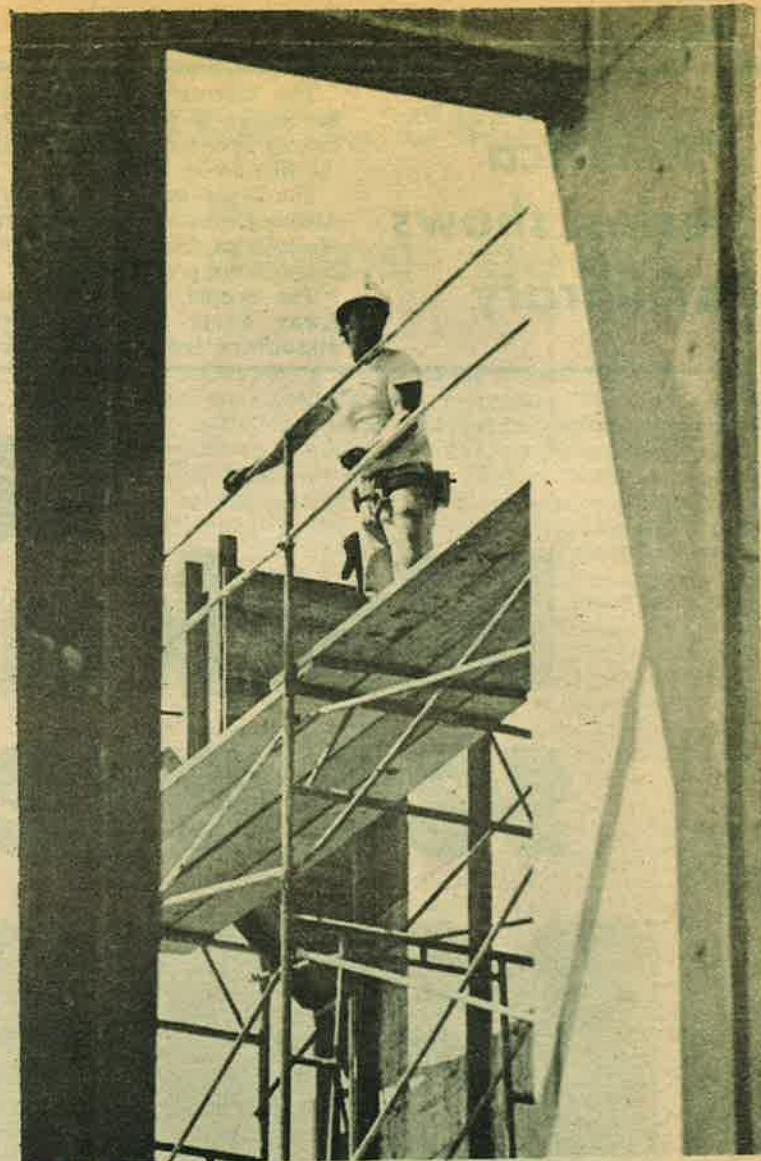
Taking Shape A construction worker views progress of the Forum Hall building from a bird's-eye standpoint on a scaffold. More photos on page 4.
